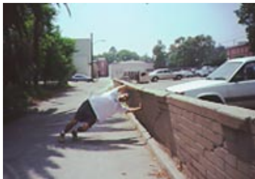
Armando Hurtado demonstrates an advanced brace retrofitting technique on the "Leaning Wall of Pasadena."
